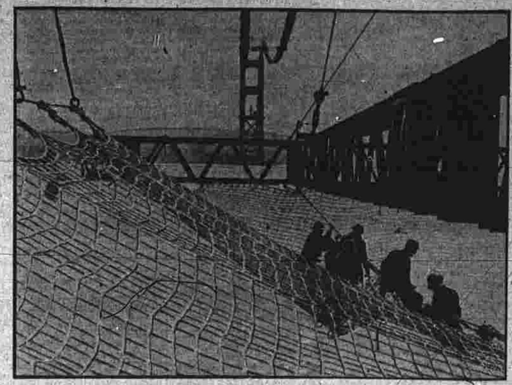
Death takes a holiday for steel workers on the gigantic bridge spanning the Golden Gate at San Francisco, since this huge life net was installed. Strung beneath the steel framework of the bridge, it is designed to catch workmen should they make a misstep on the girders towering high above the bay. The net is said to be the first of its kind to be used on construction jobs of this character.
